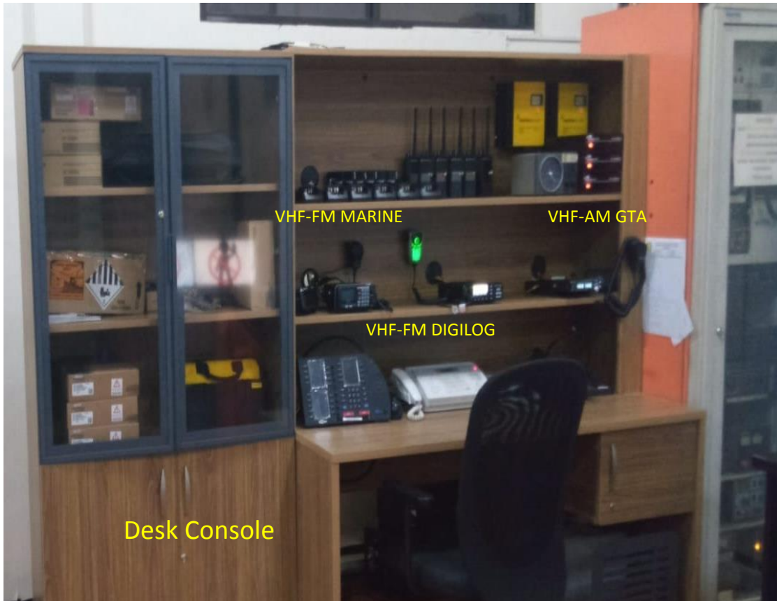
Gambar 20 Peralatan Base Communication System KPP Mataram
