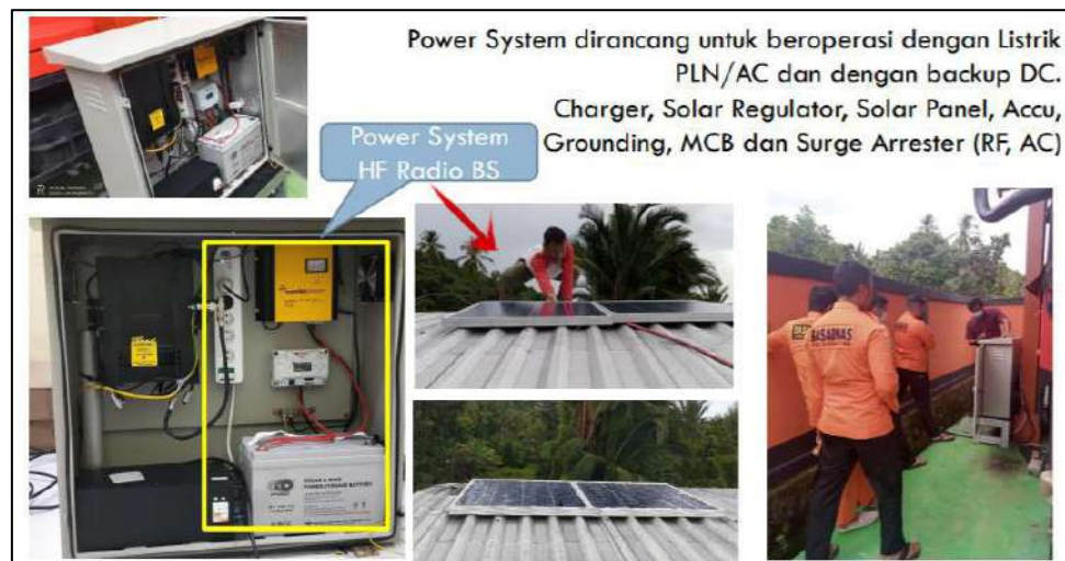
Gambar 11 - Peralatan Base Communication System
