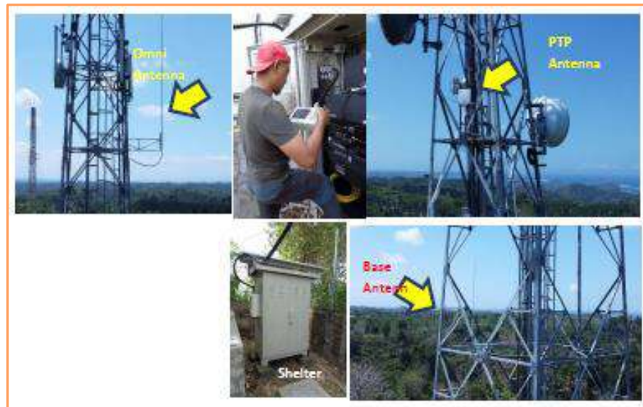
Gambar 13 - Shelter dan Antenna Tower TBG
